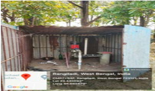
Water Supply (Pump)
